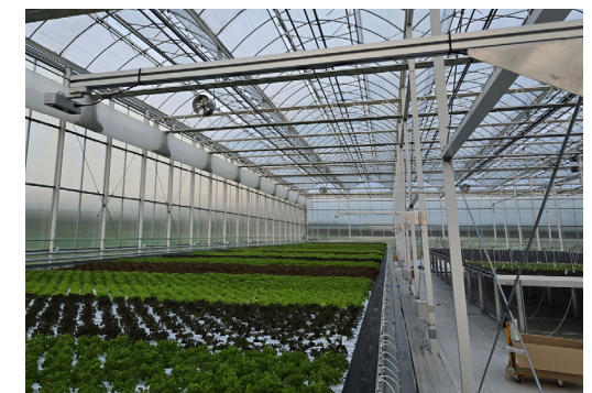
Image of Croft's Greenhouse Monitoring Equipment Installed (Source: Croft)
